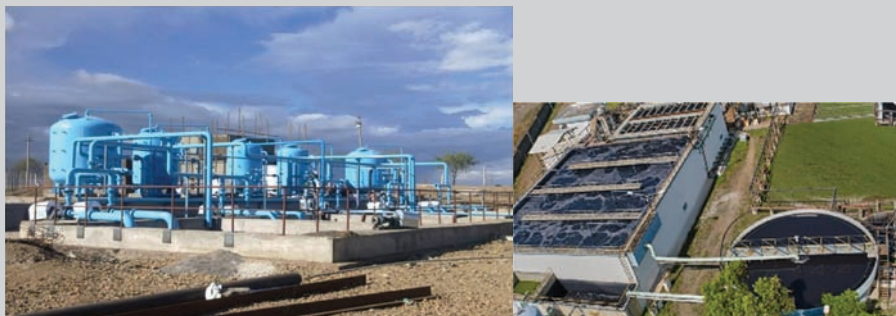
ATE Wastewater treatment plants
